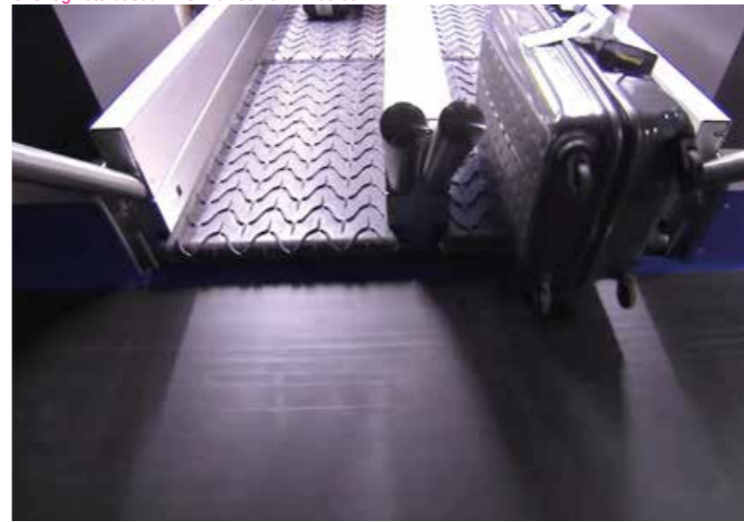
The 28 kilometre long Baggage Handling System of the Midfield Terminal will have 30 flight-build and 10 reclaim carousels, as well as 4,800 positions in its Early Bag Store.
