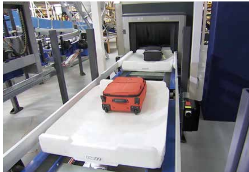
The Baggage Handling System can process up to 19,200 bags per hour with an average transfer in-system time of only 9 minutes.
