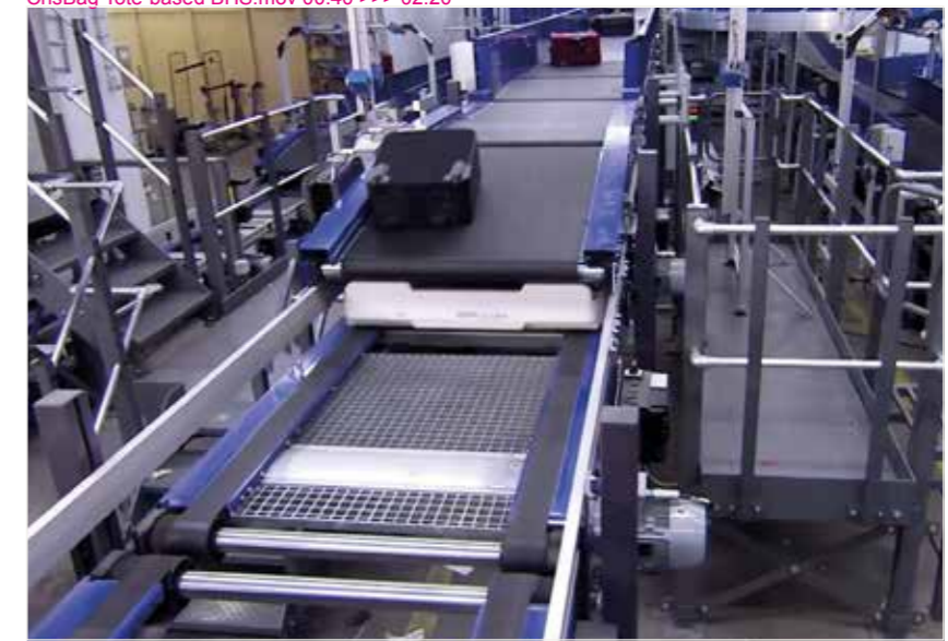
Bags will travel in the system at a speed of 25km/h, and will be screened inline at a remarkable speed of 20 bags/minute (per screening machine).
