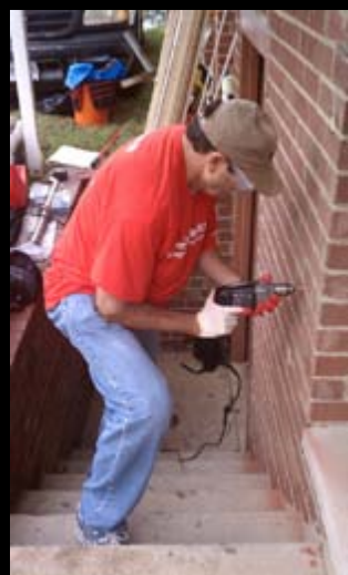
Volunteer, right, installing a handrail for exterior steps to prevent falls and broken bones.
