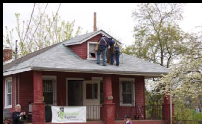
Roofers busy laying down new front porch roof at the home of a 69 year old woman, in Ward 7, who was forced out of her home because of the deplorable conditions. A heartfelt thanks to Booz Allen Hamilton, especially long-time House Captain Wade Leonard, for taking on this most challenging, yet rewarding project.
