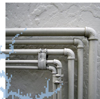
Water moves through three miles of PIPE
