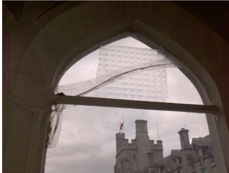
(Fig 3.2- Cracked glazing)
