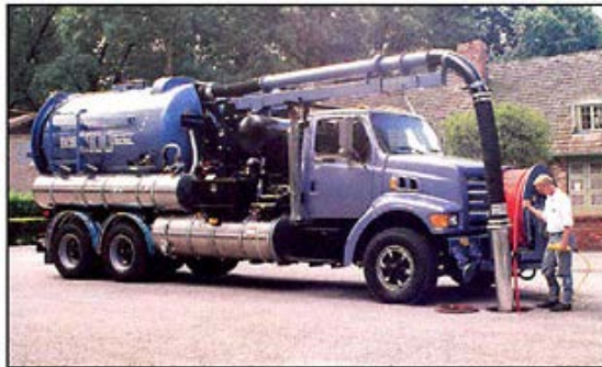
Figure 13: Catch basin cleaning (Robert Pitt, University of Alabama)
