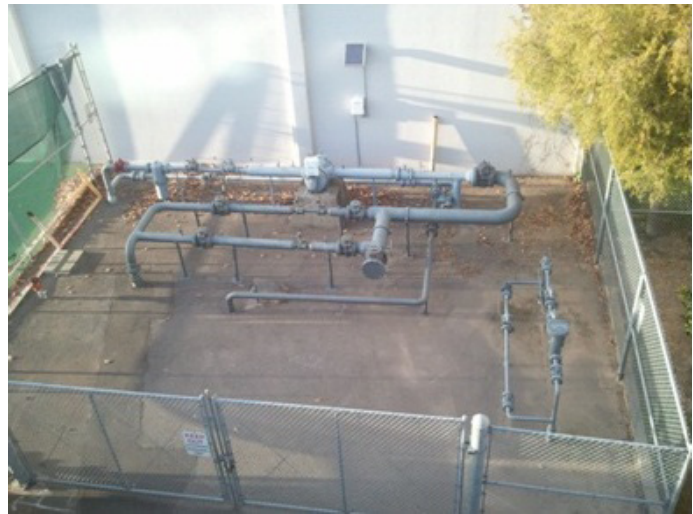
Central Campus Gas Meter
