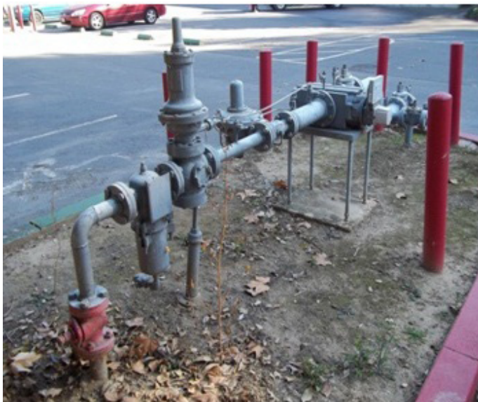
Residence Hall Gas Meter
