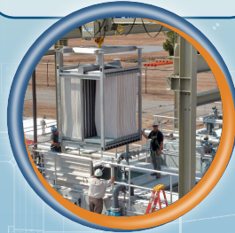
Membrane Bioreactors for Reclaimed Water Rio Rancho, New Mexico
