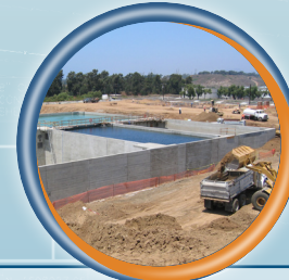
Southern Region Tertiary Treatment Plant at Marine Corps Base Camp Pendleton Oceanside, California
