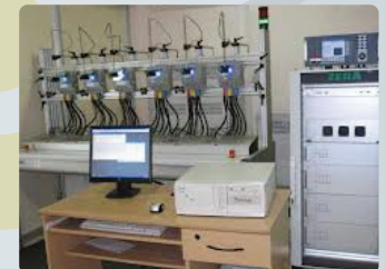
ON SITE KILOWATT HOUR CALIBRATION
