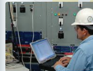
SIMULATION AND CALIBRATION OF METER, RELAY & CONTROLS
