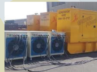
LOAD BANK TESTING
