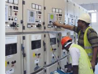
PARALLELING PANEL TROUBLESHOOTING, TESTING & COMMISSIONING
