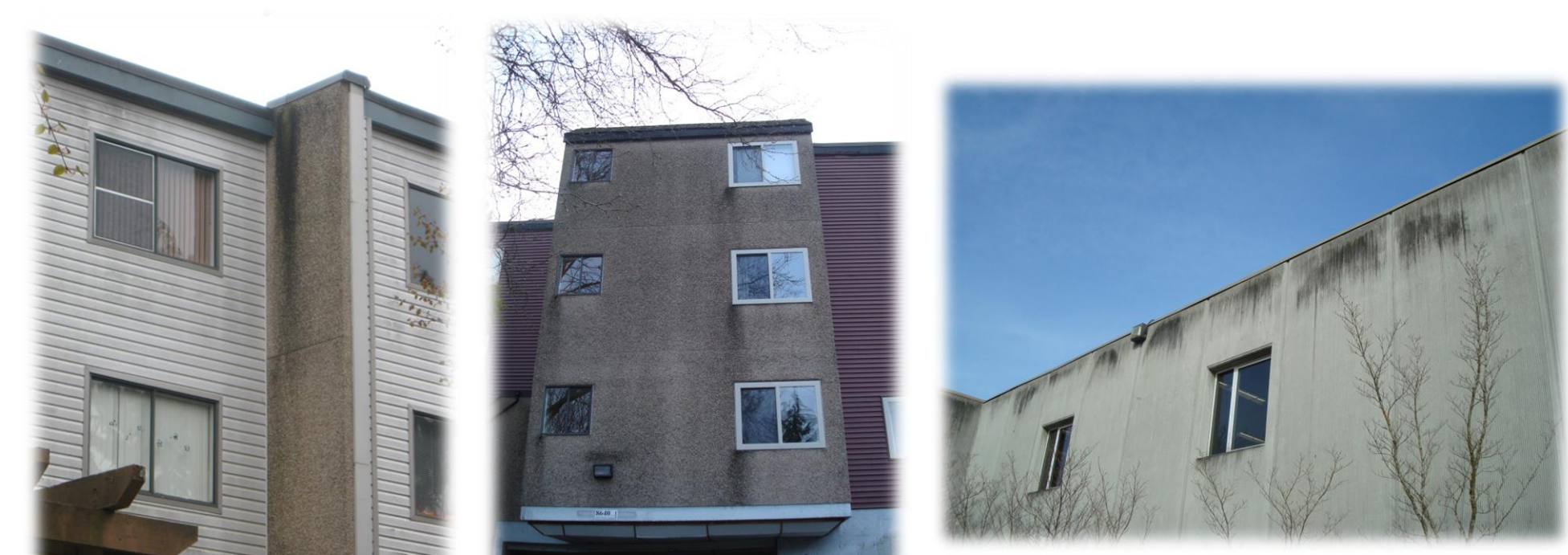
Staining & Dirt Deposition
