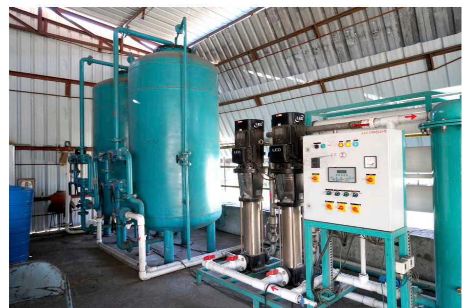
R O Water plant for Thermex Quenching system
