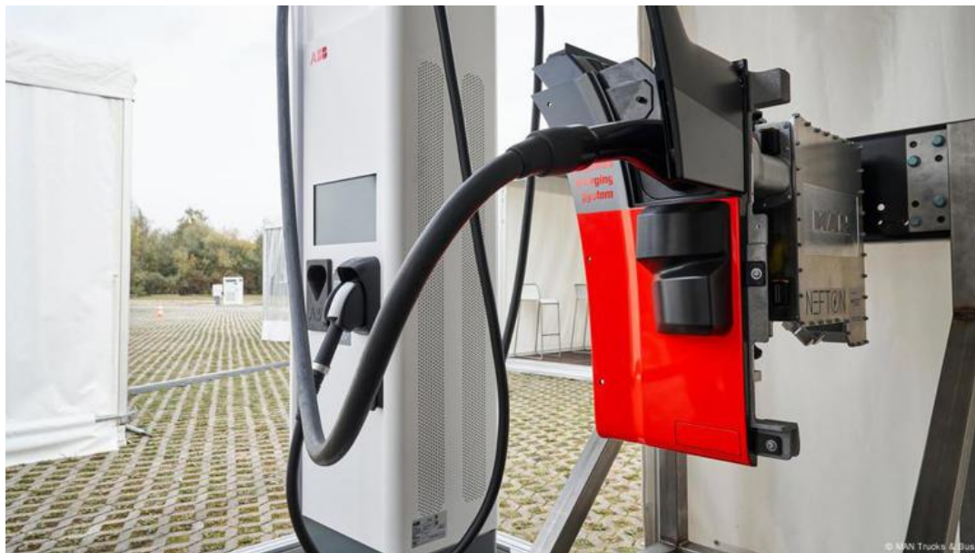
Infrastructure for megawatt charging systems would cut down charging time for trucks© MAN Trucks & Bus
