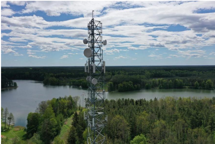
Base station (illustrative photo)
