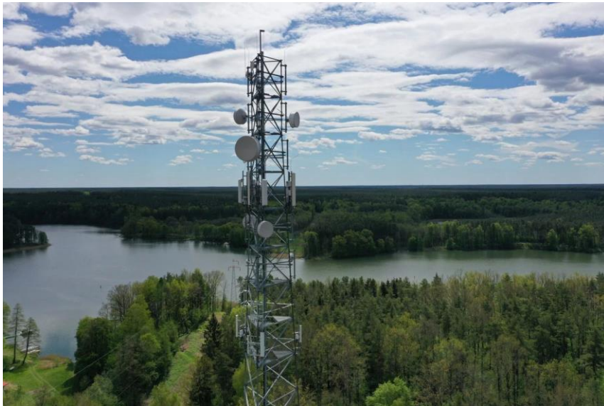
Base station (illustrative photo)
