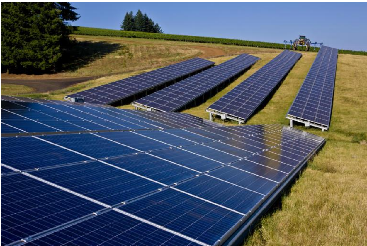
An array of solar panels, located in a vineyard at Domaine Drouhin in the Dundee Hills, is viewed on July 25, 2012, near McMinnville, Oregon. The state will soon be home to the largest solar power facility in the U.S.. Getty Images© Getty Images
