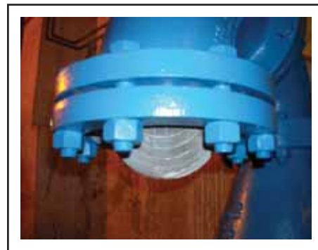
VentSafe® Security Cage Installed on Vent Pipe
