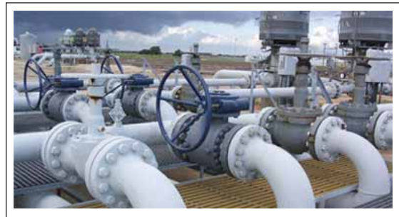
Salt Dome Brine & Gas Pumping Station
