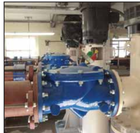
Crystal Springs Pump Station Roanoke, VA
