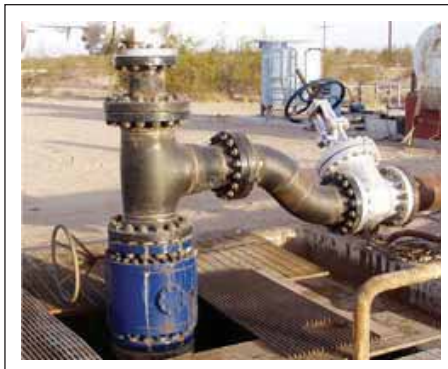
Master Valve Geothermal Brine
