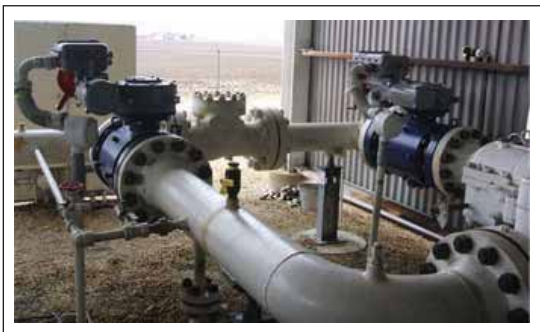
Crude Oil Pumping Station Pig Launcher/Receiver
